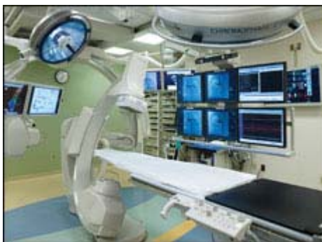
Equipment placement within the IR room is crucial.
